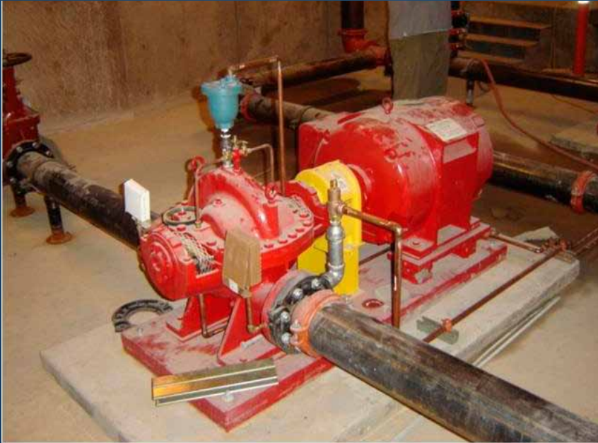
Inlet from tank @ R
